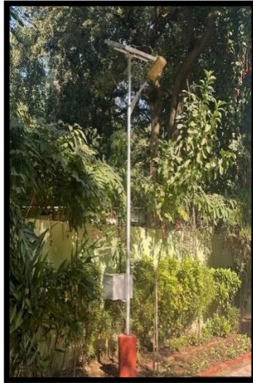
Solar Light in Boys Hostel
