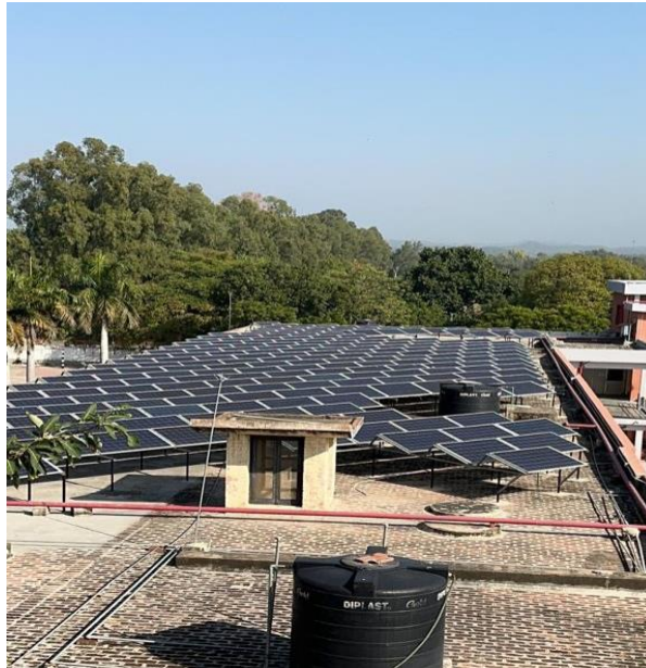
Solar Panels on the rooftop of Boys Hostel of the College
